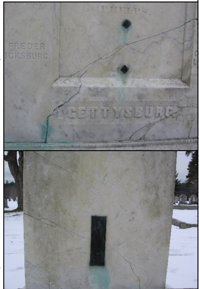
The cracks and losses are alarming. If not repaired soon, the stone will be irreparably damaged.
